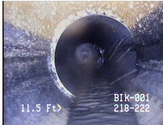
12.0 STATION DEFECT Transition from concrete to ABS
